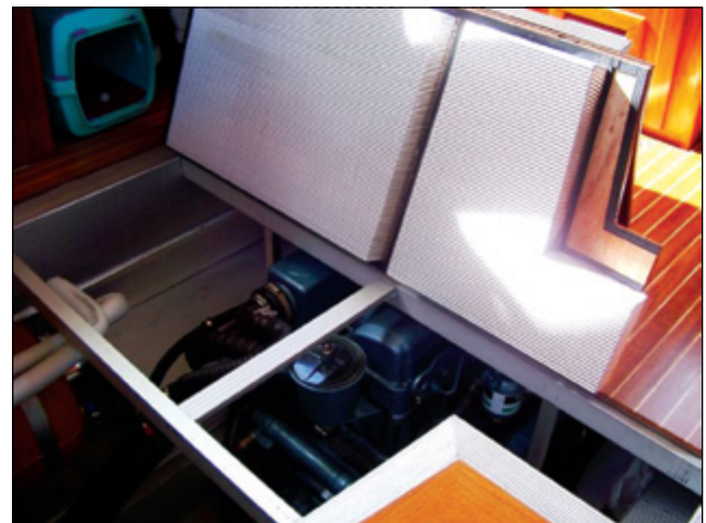
Figure 2. MPP absorbers used in engine compartment of a boat.
